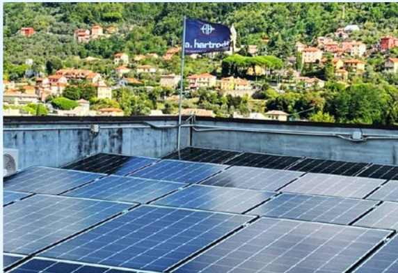
Using solar energy in the storage area of our branch in Genoa.
